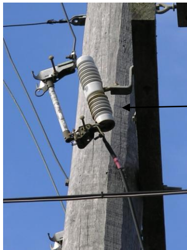
← Enlarged photo of a Drop out fuses
