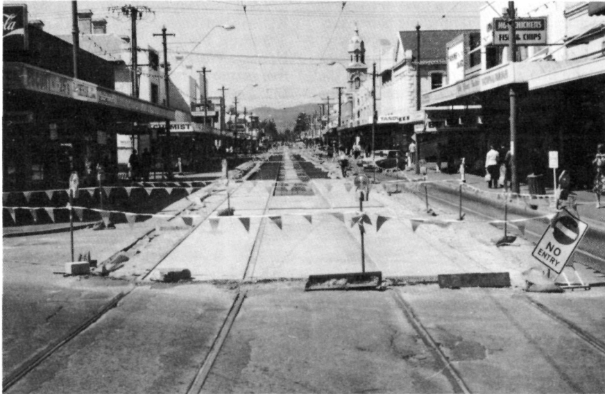
Track reconstruction in mass concrete. Jetty Road, Glenelg looking from Mosely Square in October 1982. P. Shillabeer
